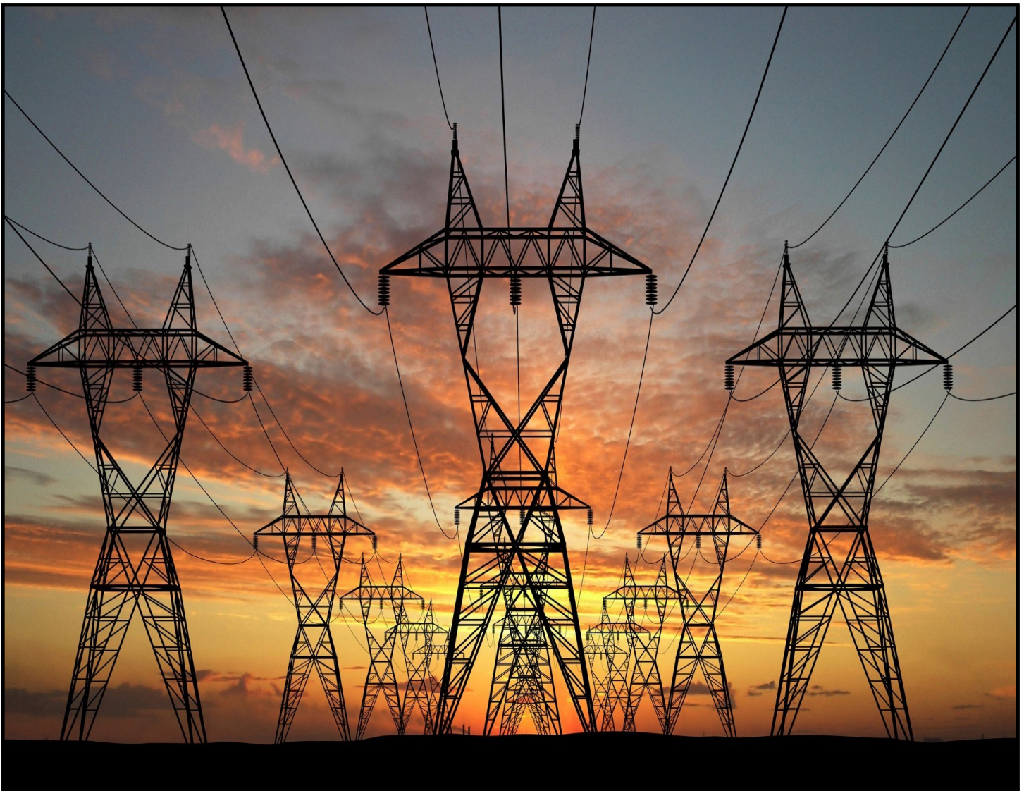
High Voltage Transmission Lines
