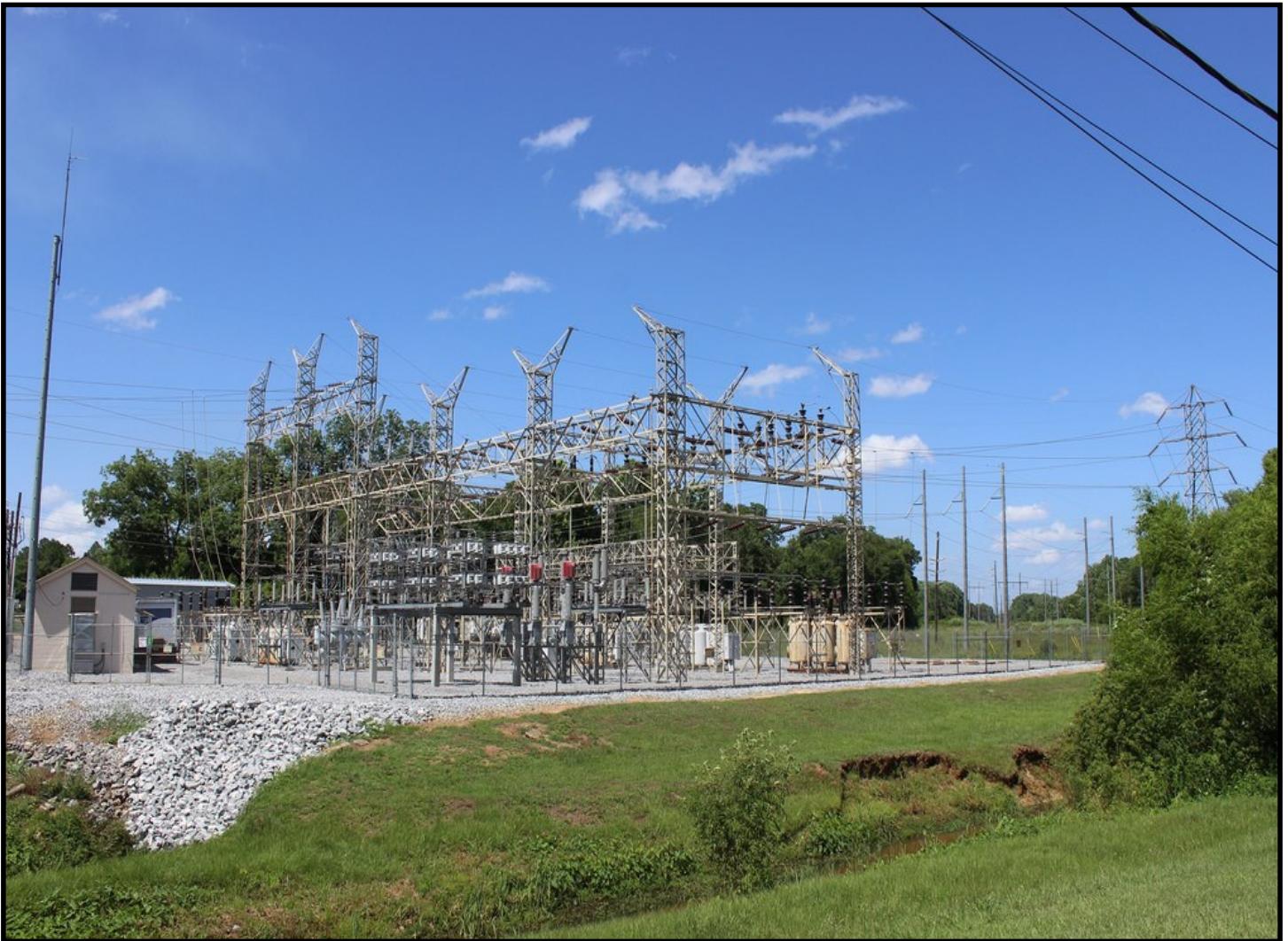
Georgia Power Substation
